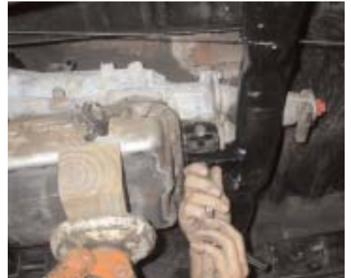
20 Hot Rod Assembly Line built the rear cross member. Tom is going to run the Dakota electric speedometer & gauges, so the S & P harness will supply a wire to run the speedometer
