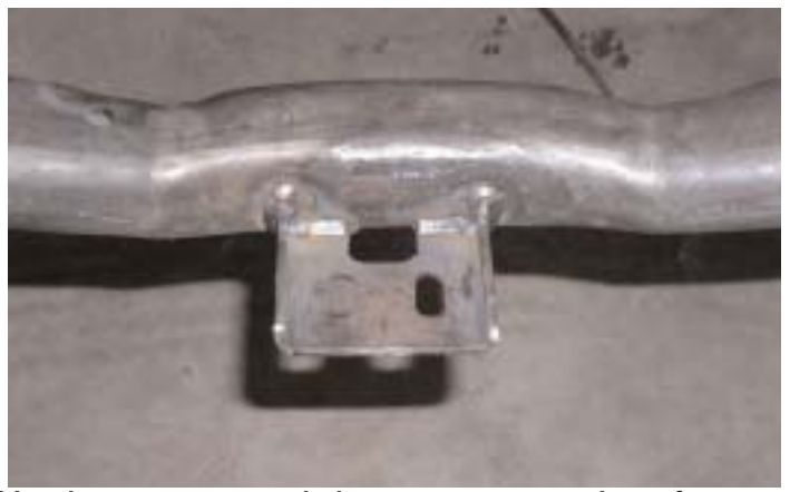
We then removed the cross member from the vehicle and finished welding the transmission mount support to the cross member.
