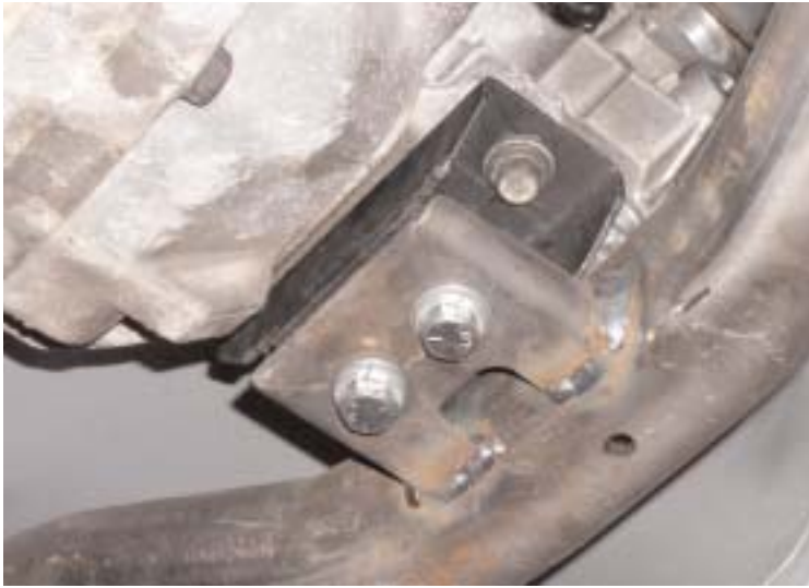
We reinstalled the cross member for a final check to insure a proper fit before detailing the finished product. Everything fit perfect.
