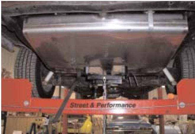
With the tank in position, we checked for clearances and filler neck alignment before tightening the stainless straps that are supplied with the tank.
