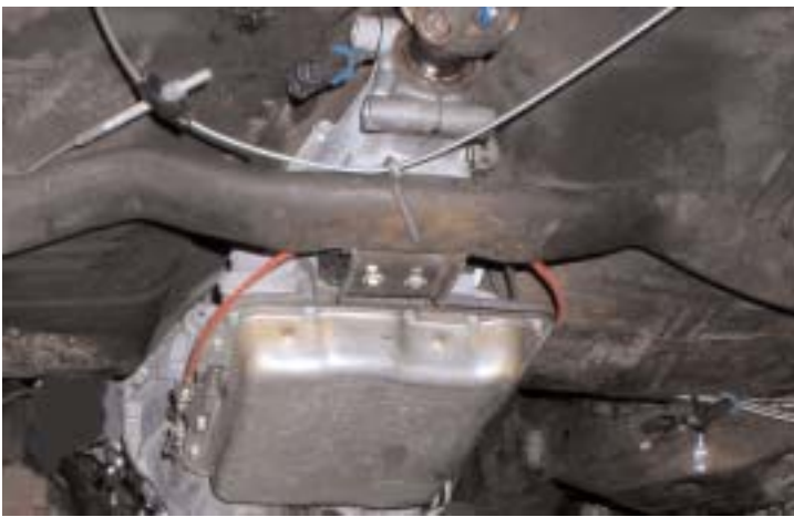
Shown above is the final installation of the 4L60E onto the original trans cross member.
